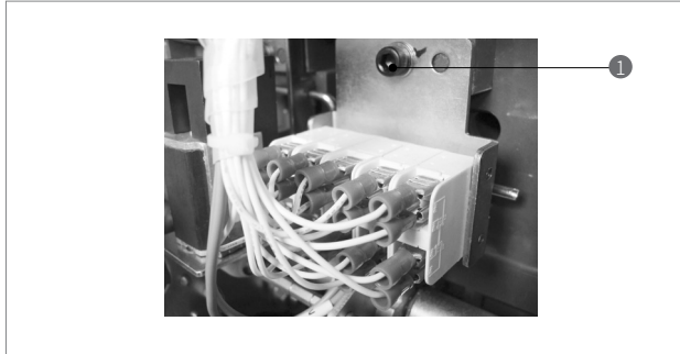
Fig. 14. Aux. switch general view
